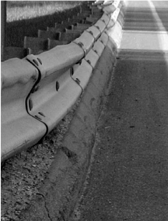
Figure 2. Sloping curb installed flush with a strong-post W-beam guardrail on a 90 km/h two-lane rural roadway in Maine.
