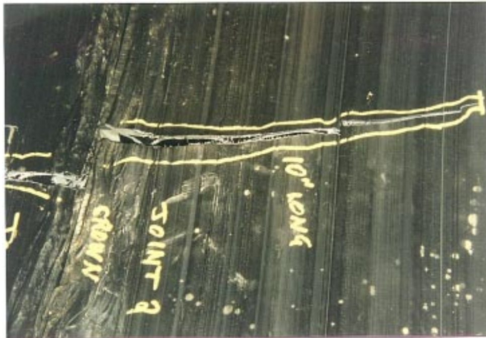
Figure 2 – A longitudinal crack in the pipe
