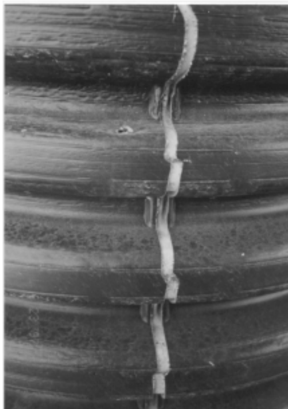
Figure 2 – A close view of the longitudinal crack along the air channel of the pipe
