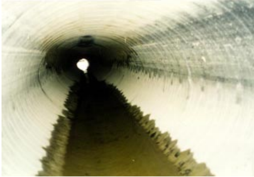
Figure 1 – a general view in the interior of the pipe at Site K
