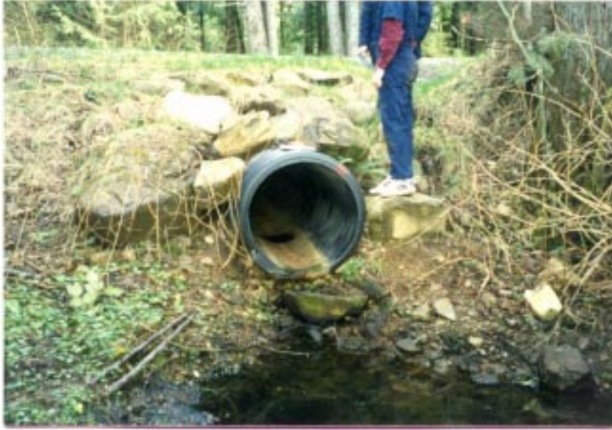
Figure 1 – A view on the outlet section of the pipe at Site V
