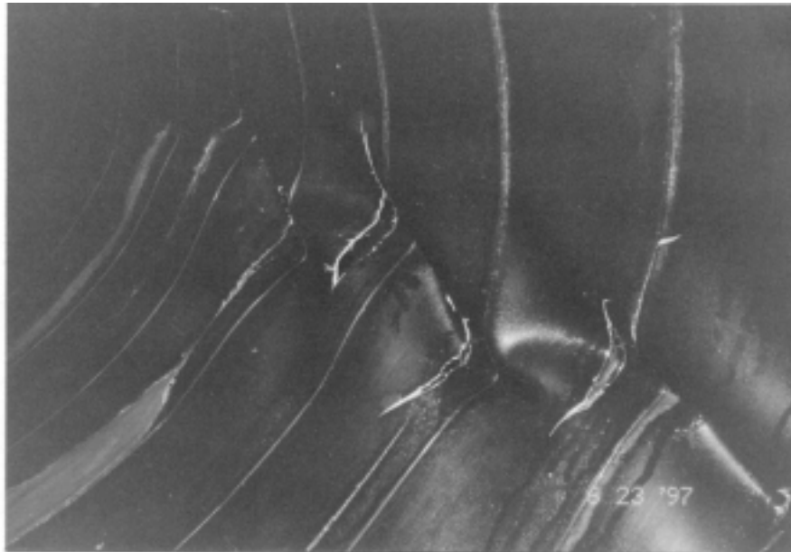
Figure 1 – Buckling and cracking in the liner of the pipe
