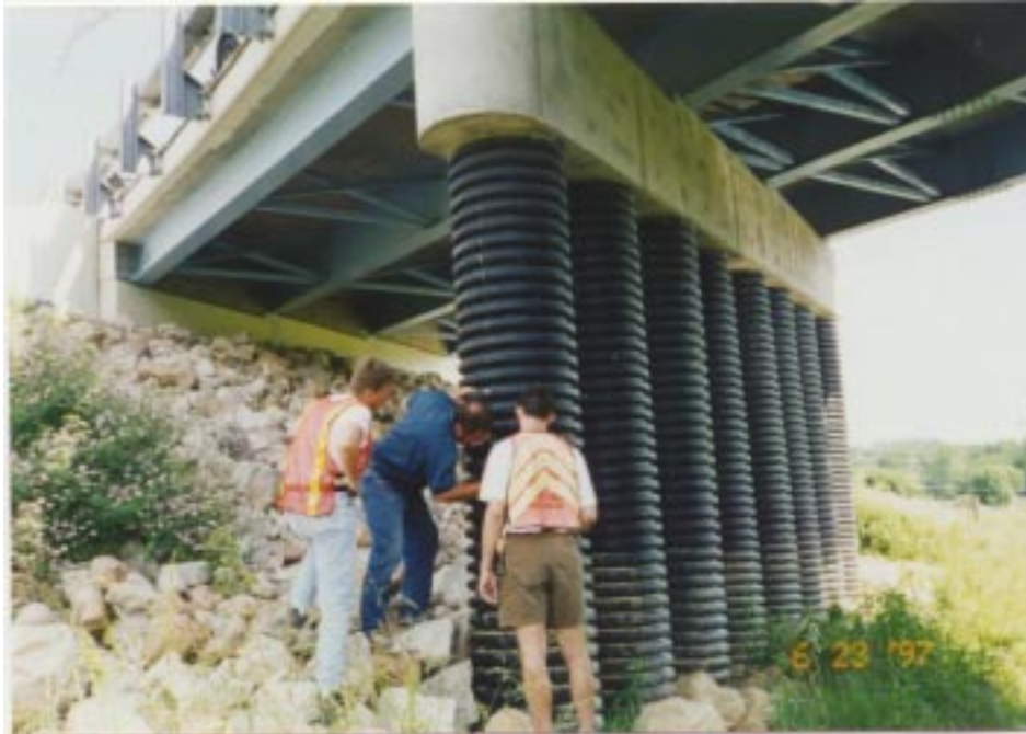
Figure 1 – A view of the eight concrete columns with pipe as the formwork
