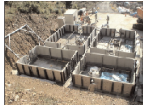
Japan's SPER system for rapid construction of bridge piers uses precast concrete panels as structural elements and formwork. (Photo courtesy Sumitomo Mitsui Construction Co.)
