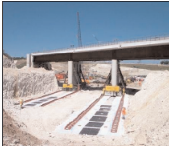
Skidding a bridge into position is one time-saving installation method used in Europe. (Photo courtesy Mammoet Corporation)
