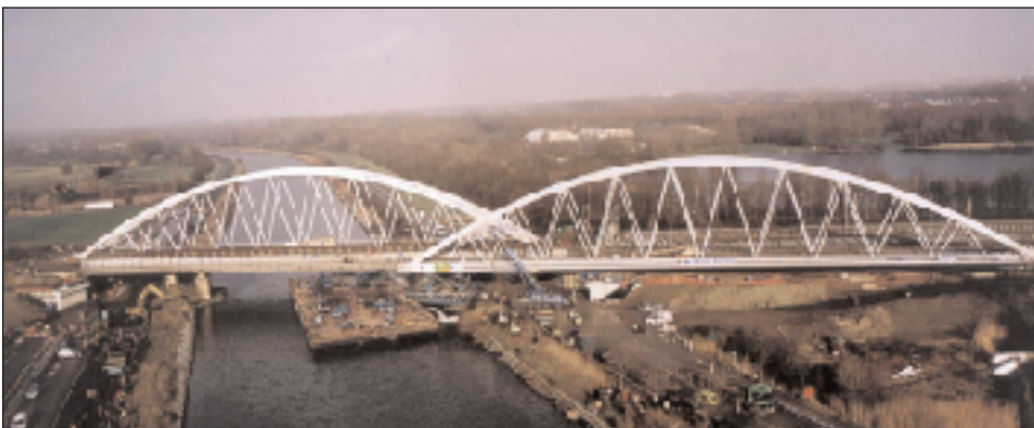
Large bridge components are moved into place with self-propelled modular transporters, or SPMTs. (Photos courtesy Mammoet Corporation and Sarens Group)
