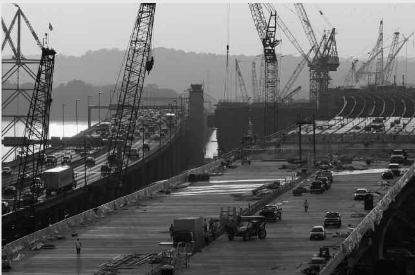
The draw spans, or bascules, of the new Woodrow Wilson Bridge, near Washington, D.C., feature eight opening leaves composed of more than 14 million pounds of steel.
