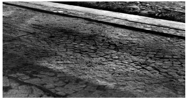
FIGURE 17 Failure of block pavers after 9,000 cycles of 40-kN loading. Note the amount of sand that has been pumped from under the granite blocks (Sharp 2001).
