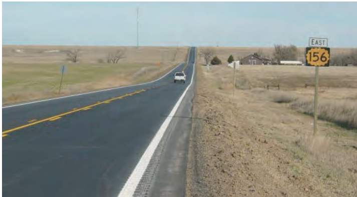
After improvements along K-156 in Hodgeman County, the benefits include a wider shoulder, rumble strips and a gentler side slope.
