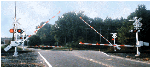
Figure 1 Typical 4-quadrant gate
