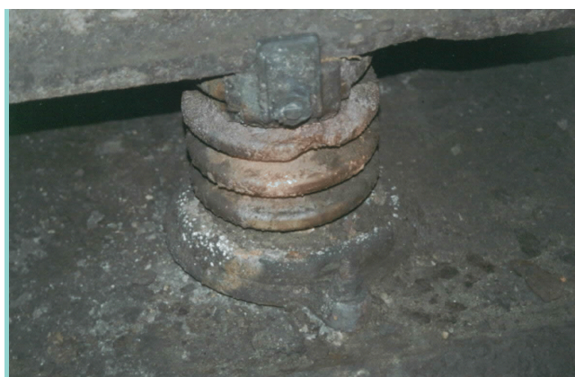
DIRTY INSULATOR AT WMATA 8/16/2001
