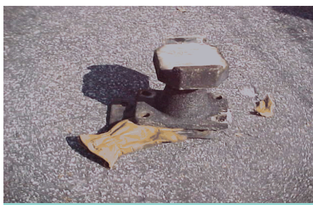
BURNT INSULATOR AT MARTA
